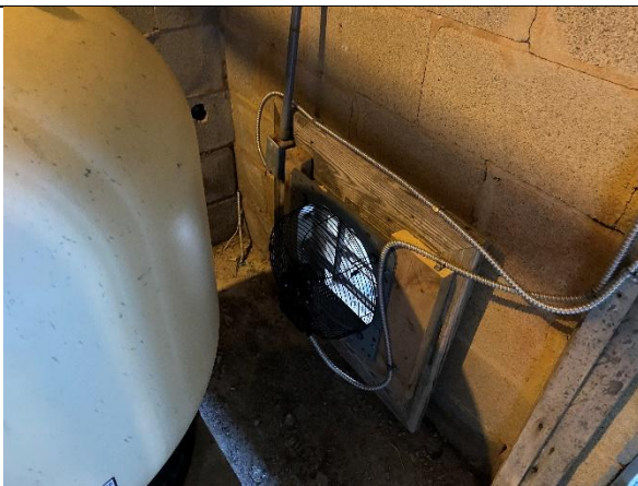
Figure 53 Mechanical Room Exhaust Fan
