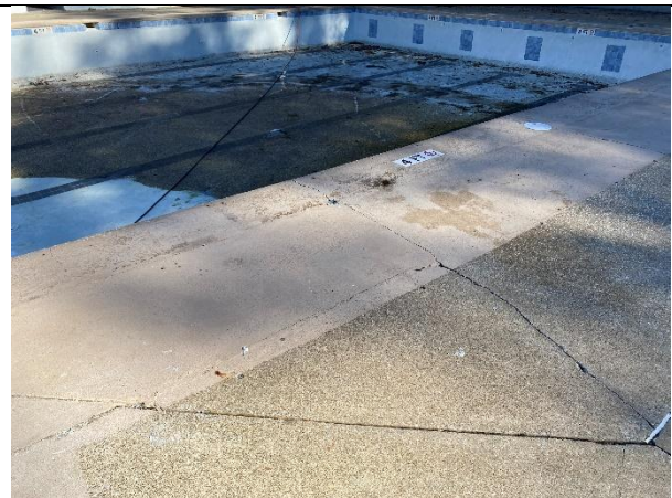
Figure 22 Pool Deck Cracking
