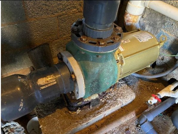
Figure 43 Pool Recirculation Pump
