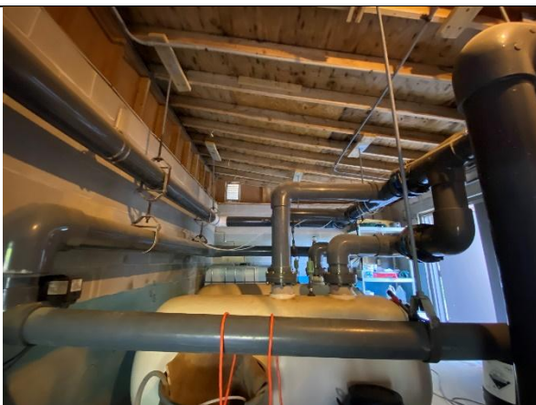
Figure 47 Pool Recirculation Piping
