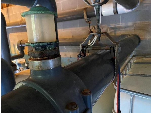
Figure 37 Corrosion on Pipe Supports
