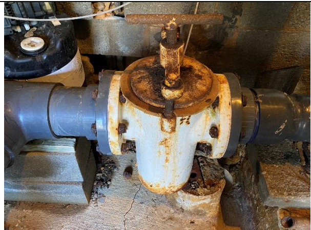
Figure 46 Pool Strainer (Corrosion)
