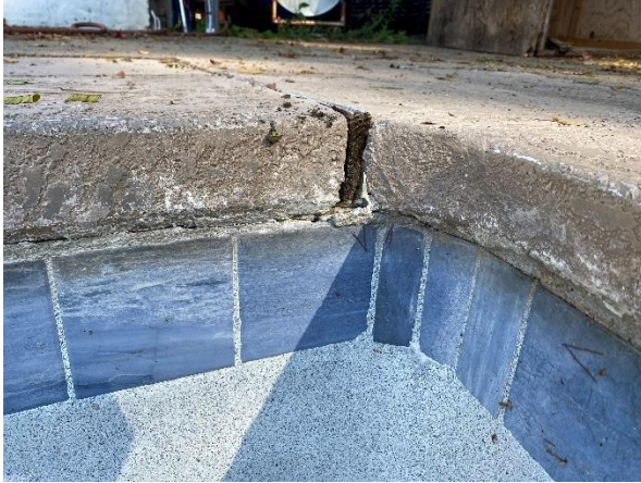
Figure 13 Separation in Coping Stone
