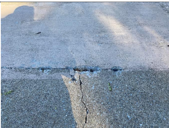
Figure 17 Cracking in Pool Deck
