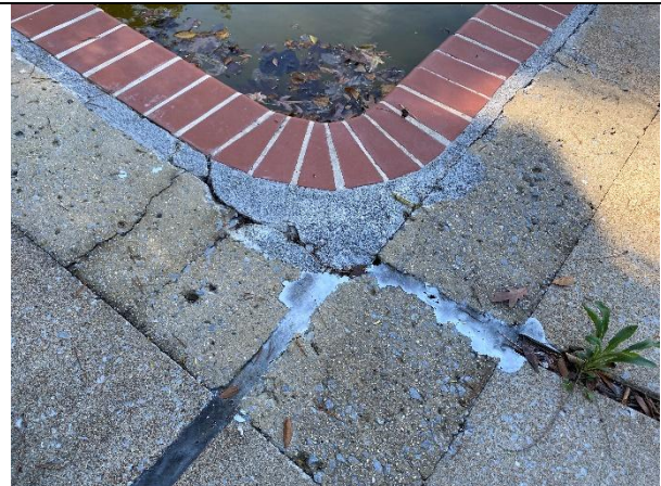
Figure 58 Cracking Around Pool Perimeter
