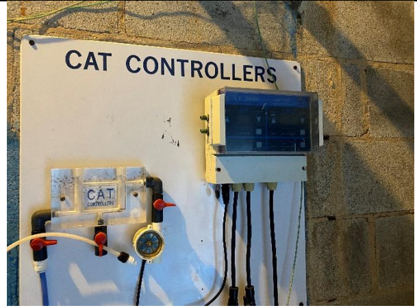
Figure 50 Children's Pool Chemical Controller
