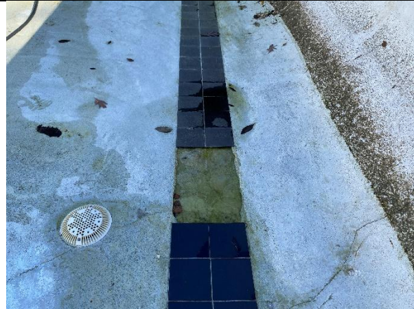
Figure 19 Missing Lane Line Tile
