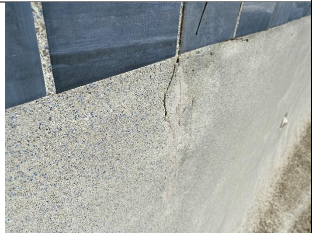
Figure 16 Vertical Crack in Pool Wall
