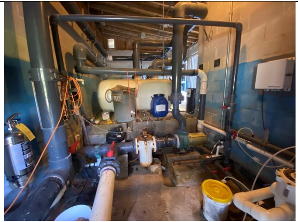
Figure 34 Pool Mechanical Room
