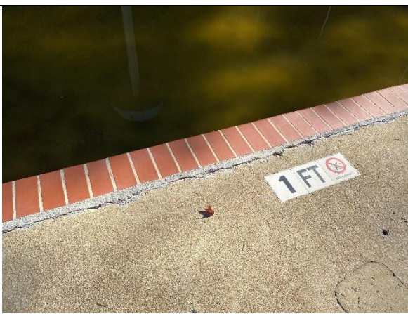
Figure 59 Separation (Coping and Deck)
