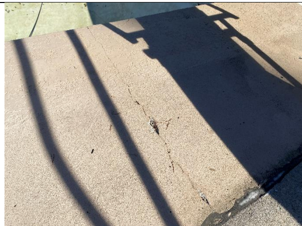
Figure 21 Cracking in Coping Stone
