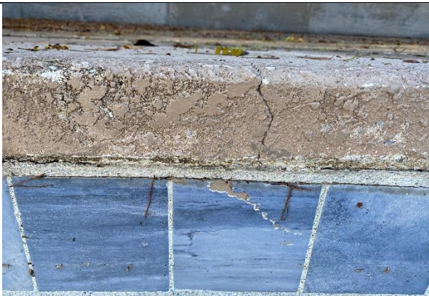
Figure 15 Crack in Coping Stone and Cracked Tile
