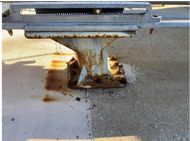
Figure 28 Diving Stand Base Corrosion
