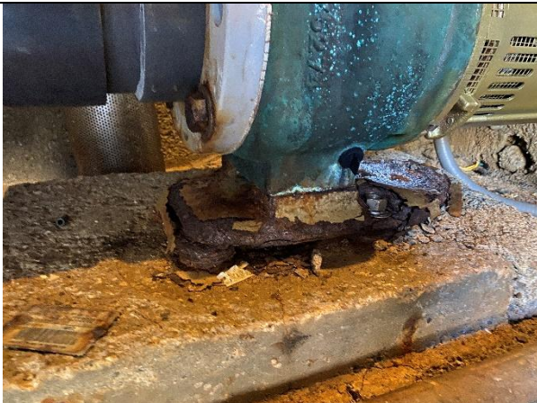
Figure 45 Corroded Pump Base Supports
