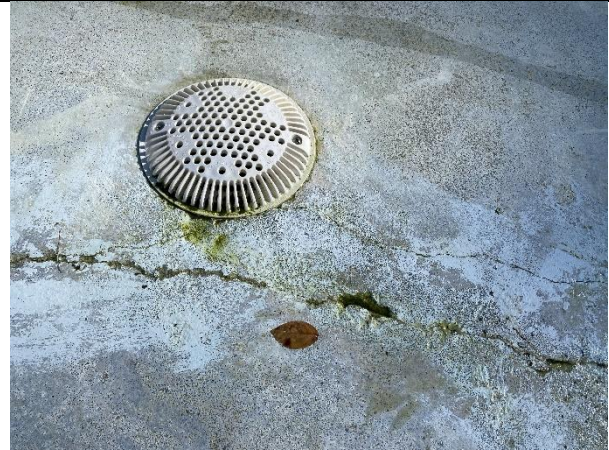
Figure 20 Hydrostatic Relief Valve and Adjacent Surface Cracking
