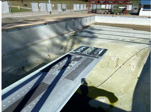
Figure 26 Delamination of Surface on Duraform Diving Board
