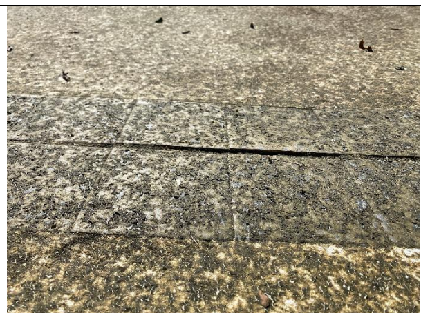
Figure 24 Missing Grout in Lane Line Tile
