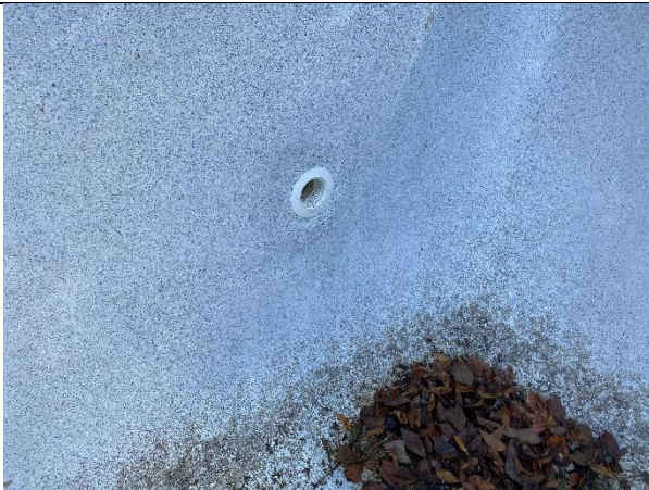
Figure 33 Return Wall Inlet (Missing Cover)
