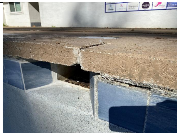
Figure 23 Cracking and Separation in Coping Stone
