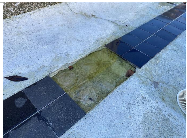
Figure 18 Missing Lane Line Tile
