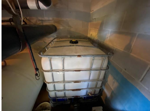
Figure 38 Liquid Chlorine Storage
