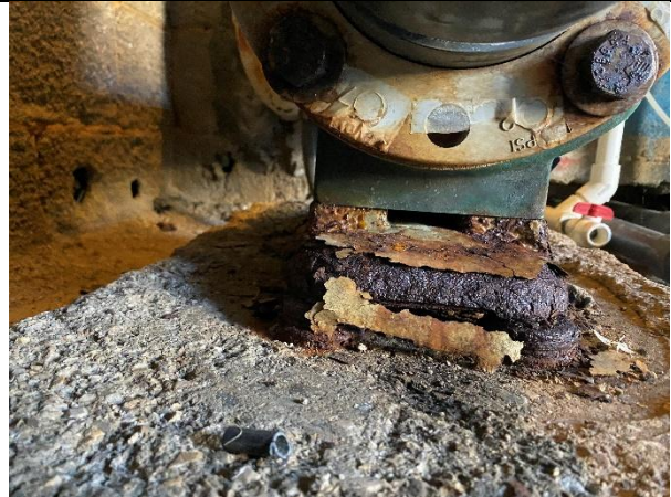
Figure 44 Corrosion on Pool Pump
