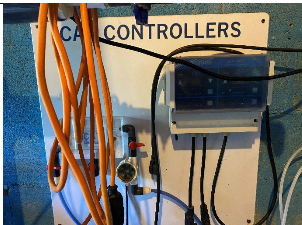
Figure 42 Main Pool Chemical Controller
