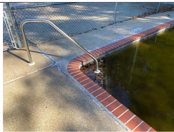
Figure 60 Cracking and Deck Separation
