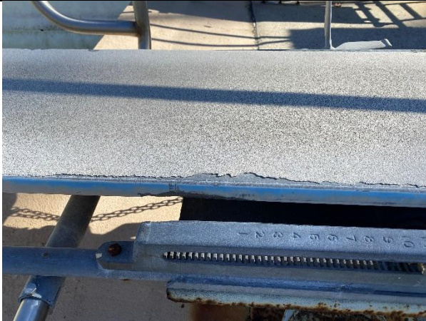
Figure 25 Delamination of Diving Board Surface
